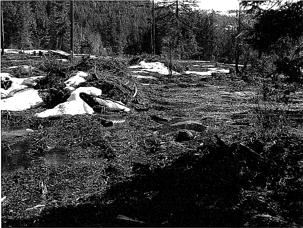
Figure 1 Clearing and grading in the headwaters of Thornton Creek on the Daniels short plat April 2008
